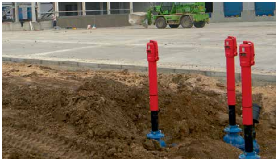
AVK series 34/00 post indicators for fire protection at FM Logistics - Petresti, Romania.
